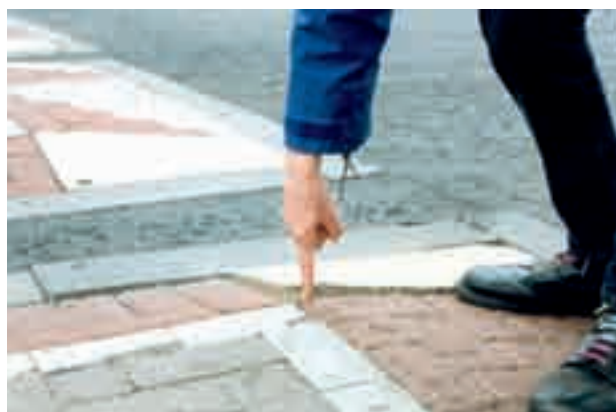
Fig. 2.8 Damage to a speed cushion
